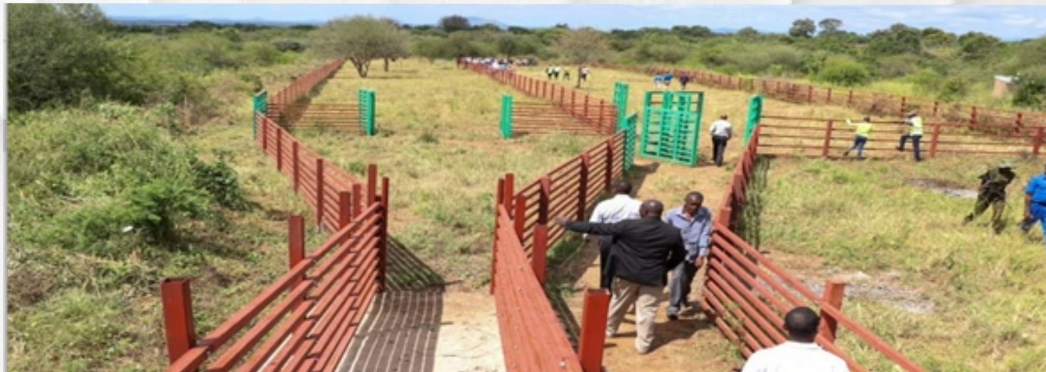
Figure 10:Ongoing Construction Kathonzweni livestock yard, the 4th largest livestock yard in Kenya
