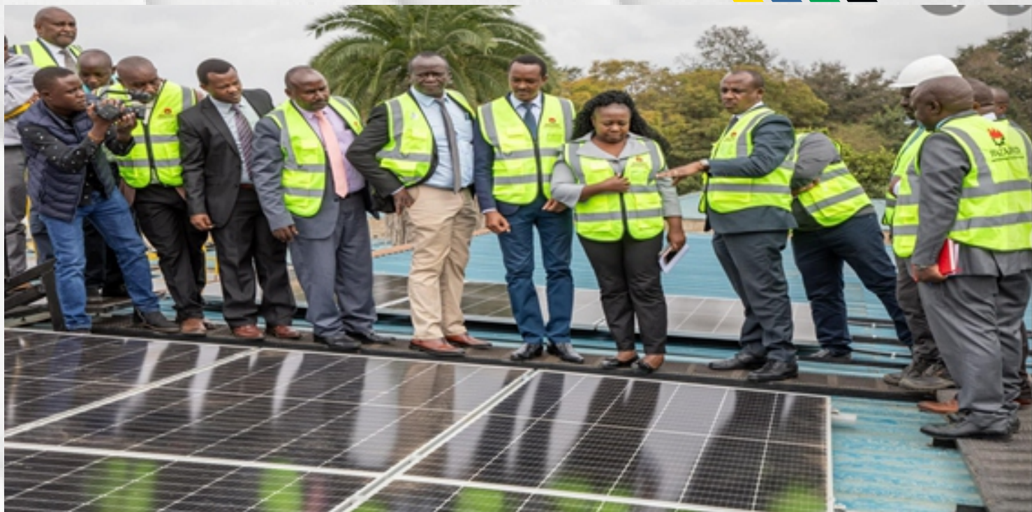
Figure 22: H.E Mutula Kilonzo Junior During The Commissioning Of Phase 1 Of Productive Use Of Renewable Energy (PURE) At Makeni County Referral Hospital
