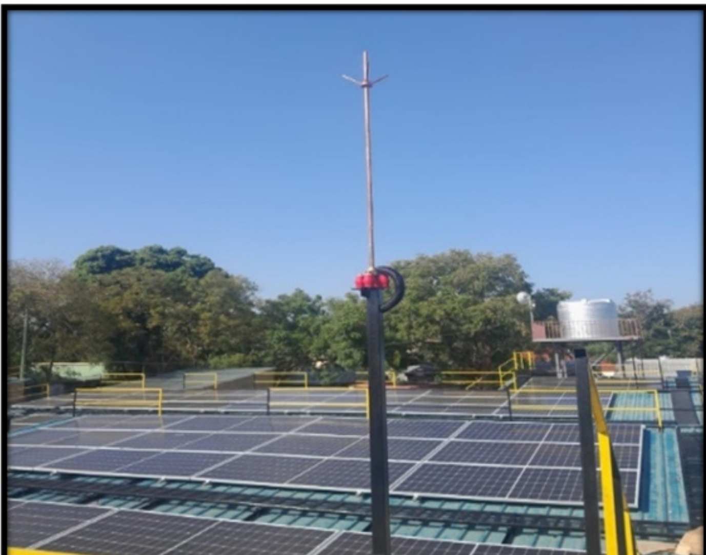
Installed Solar Plant in At Makeni County Referral Hospital
