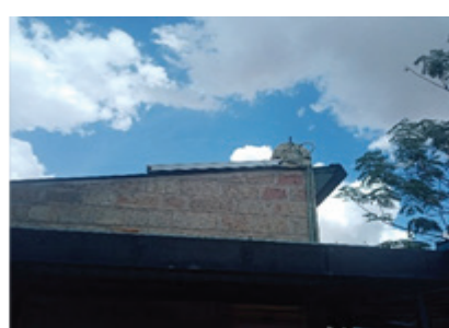
Solar water heater
