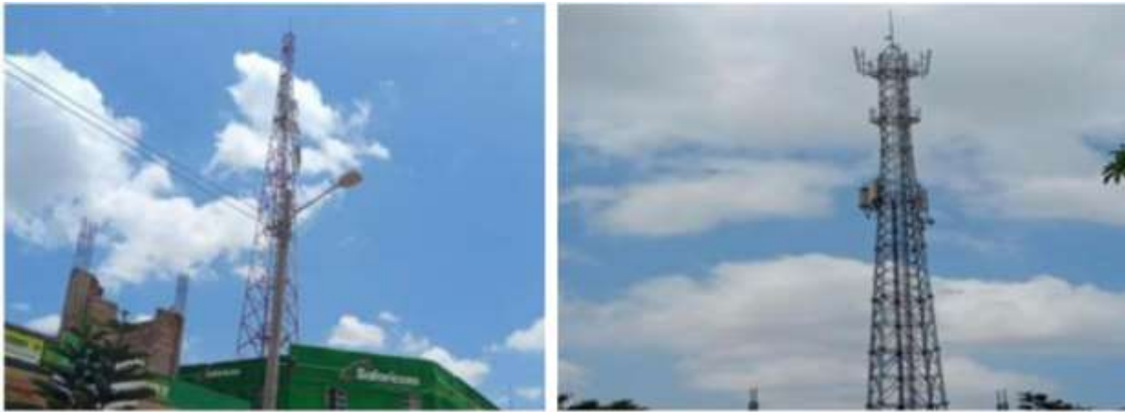
Figure 18: Telecommunication mast in Sultan Hamud and Emali Towns
