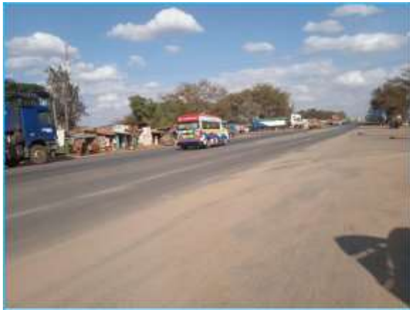
Lack of drainage channel along Nairobi-Mombasa Highway (A109)
