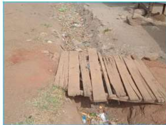
Clogged drainage channel
