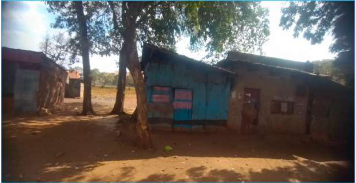
Dilapidated houses in Emali town
