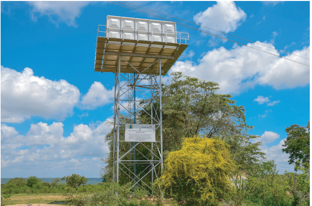
Mukelenzu Borehole storage tank
