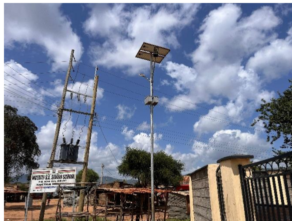
Street light at Kavuthu shopping centre
