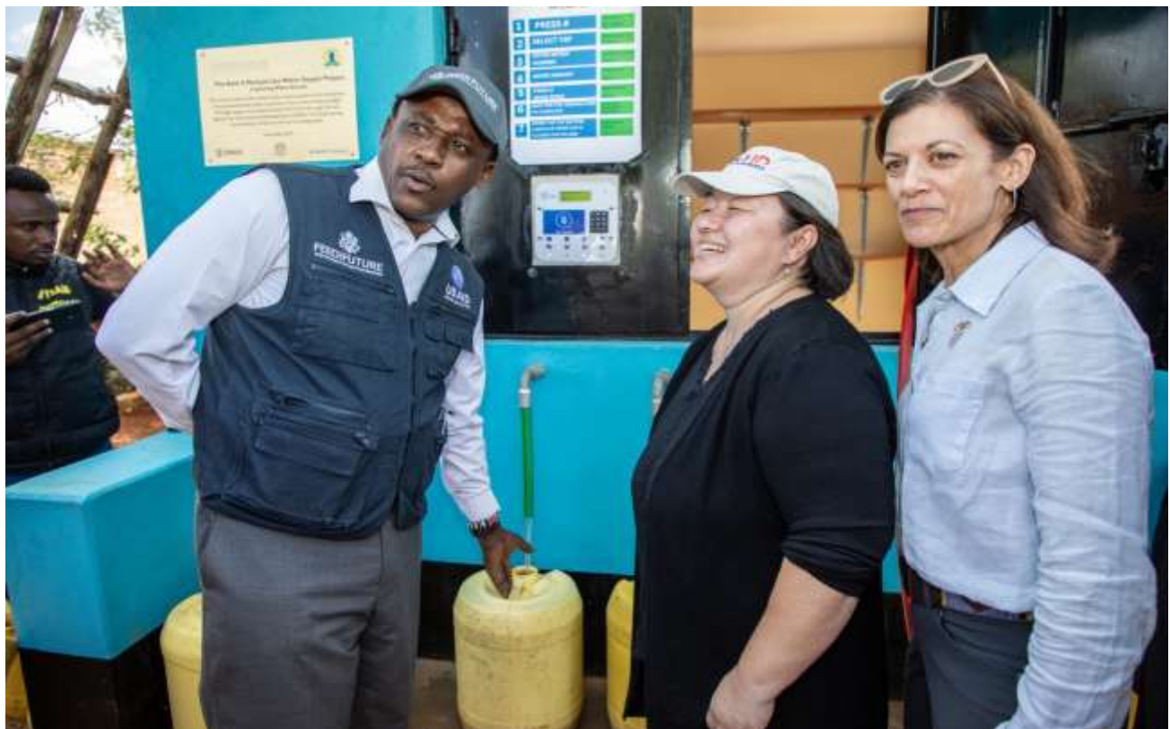
Figure 9: The Governor Makueni County (Right) together with USAID STAWI inspects the use of smart metres
