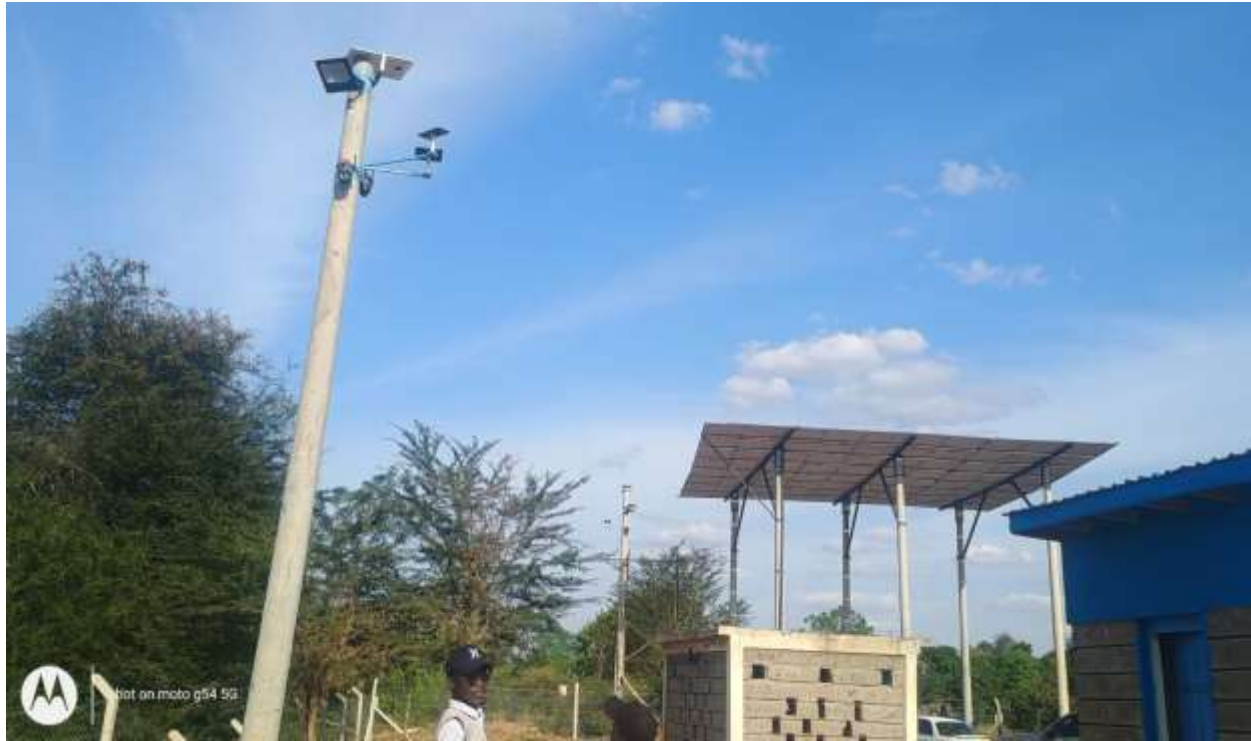
Figure 10: High Rise solar panels combined with the use of flood lights and CCTV Camera
