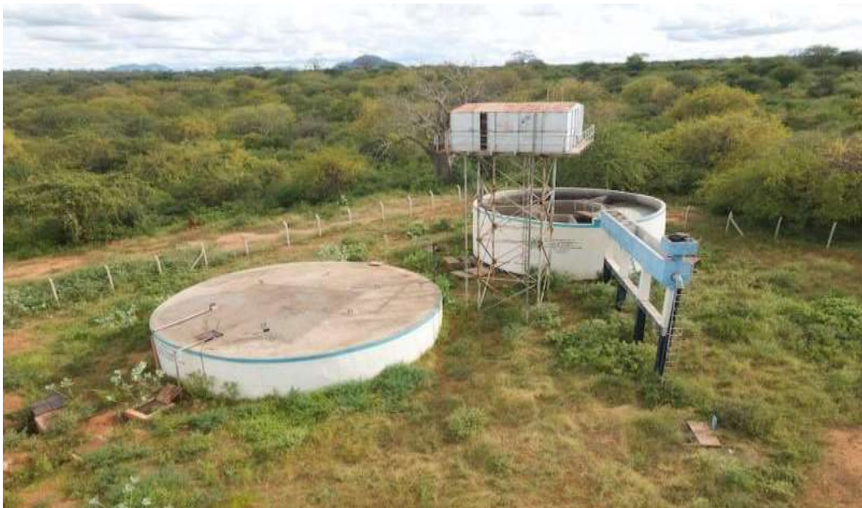
Figure 5: Athi Tunguni water treatment facility
