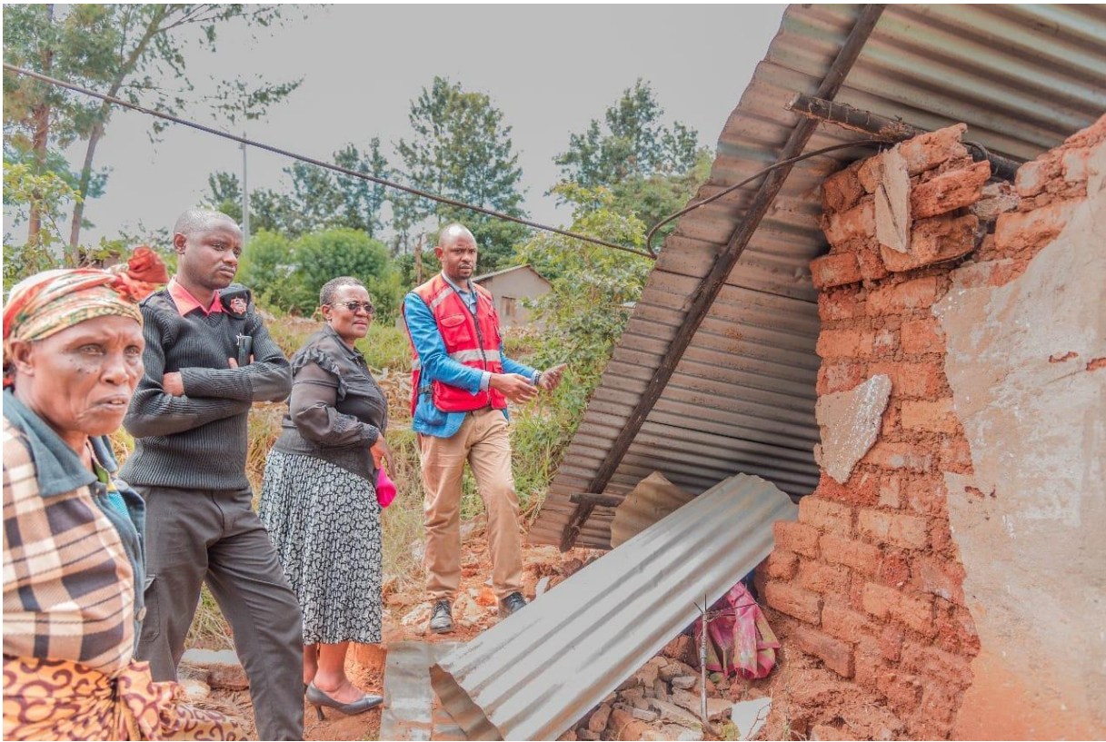
Figure 11: Effects of Flash Floods on Infrastructure
